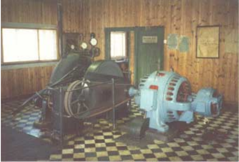
Figure 3.3. Høgfoss Elverk, Begndalen, Norway.
