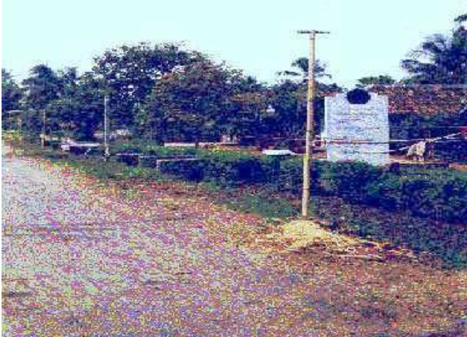
Figure 2.2. Informal (private) electricity distribution grid (220 Volt AC) with bamboo poles.
